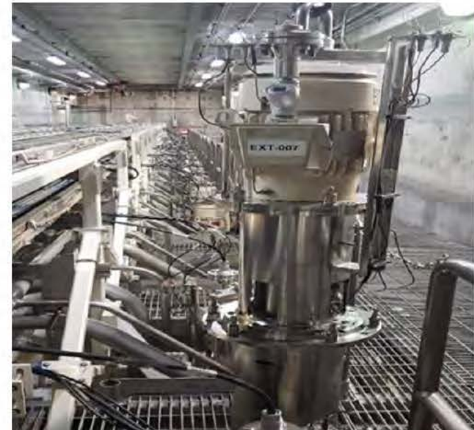
SWPF CSSX Centrifugal Contactors
